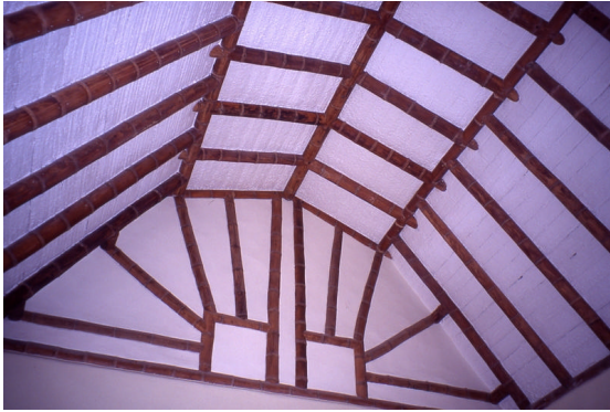
Not all of the truss needs to be visible in the final ceiling.
